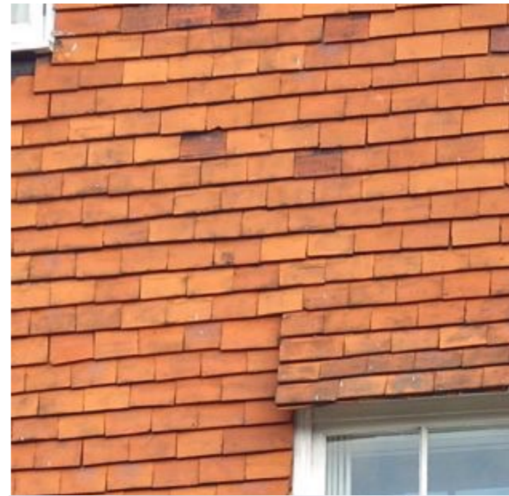
Handmade hanging tile is an historic material, but the all over covering of roof and wall and the simplicity of the edge detailing can allow for the development of a subtly contemporary sensibility in the handling of the material.
