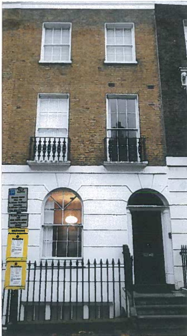
1. View of 15 Swinton Street facade showing sash window nos: W1 W2 W3 W4 W5 W6 changed from single to double glazing (see drawings 1, 2 and 3)
