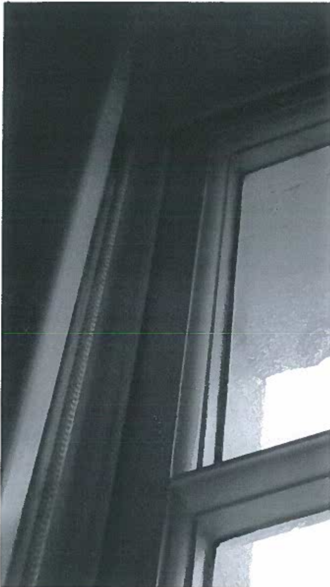
5. Detailed view of upper section of typical sash window showing top and side frame and glazing bar all with same moulding
