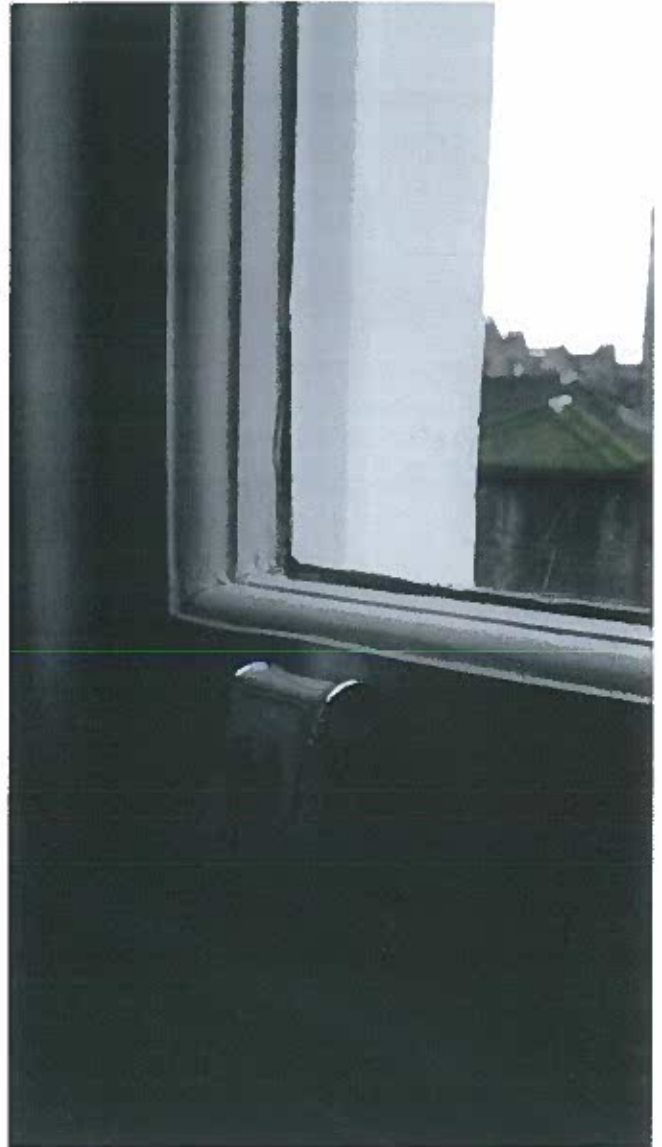
6. Detailed view of bottom section of typical sash window showing side and bottom frame with same moulding
