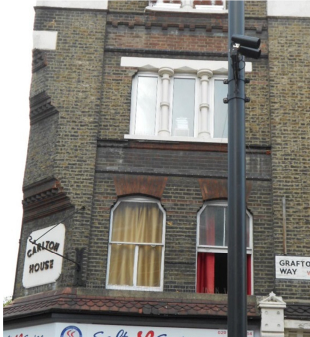
A mixture of inappropriate and poorly fitting windows
