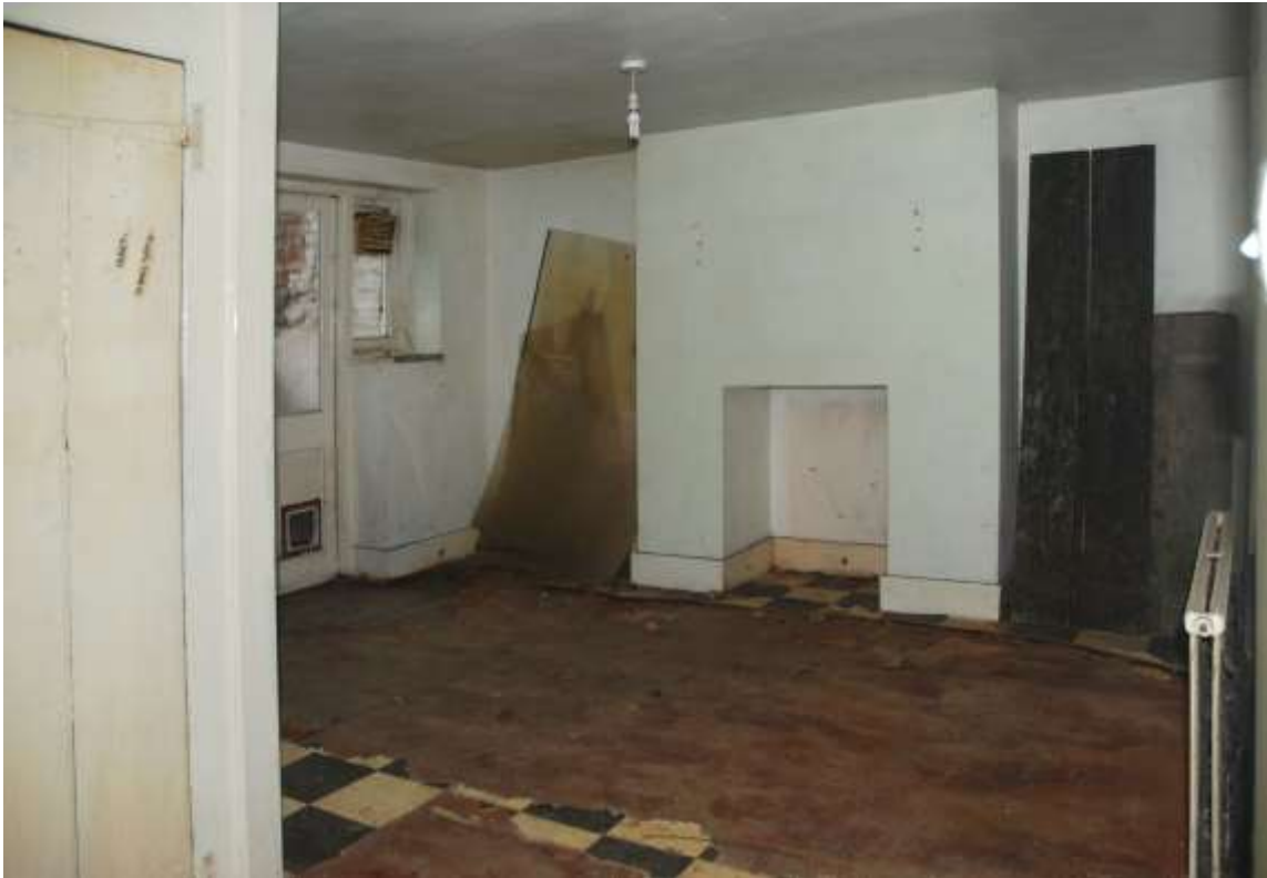
Fig.34: The rear part of the basement, showing the former fireplace on the north wall
