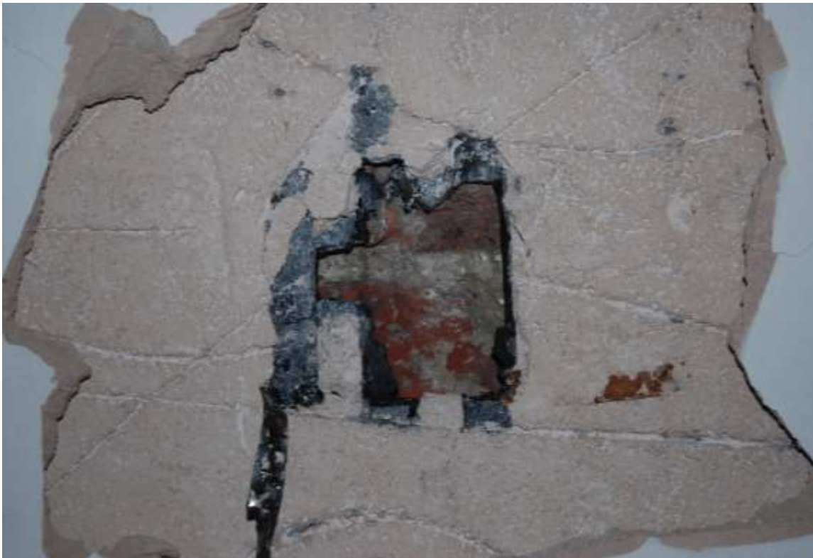
Fig.31: Detail of the dividing wall. Originally the basement walls may have been bare brickwork (or possibly previous render has been stripped off). The present covering is recent, modern plaster over a bituminous felt-type backing, as observed both here and elsewhere throughout the basement
