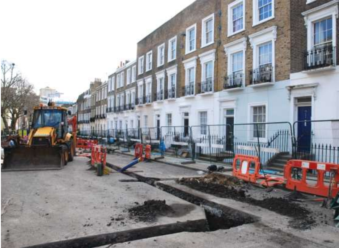
Fig.14: Water mains replacement works in progress. The present study site is in the centre of the frame (second from left of the higher terrace)
