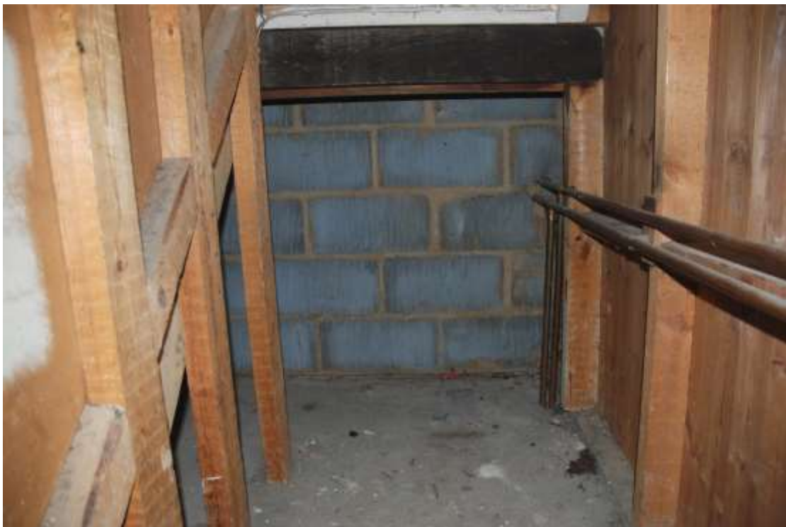
Fig.37: Interior of the cupboard, showing the quite recent structure and also a breeze block wall to the rear extension
