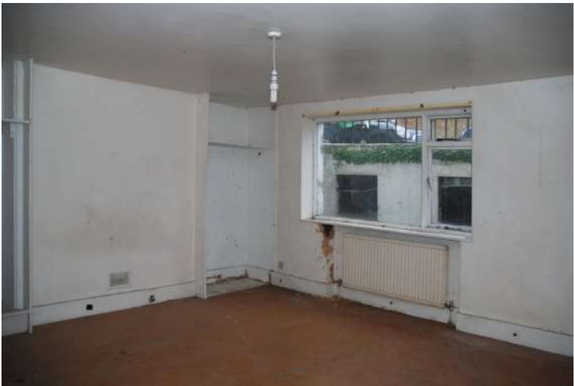
Fig.29: A further view of the front of the basement, the base of the chimney stack (& possible former fireplace) to the left of the frame
