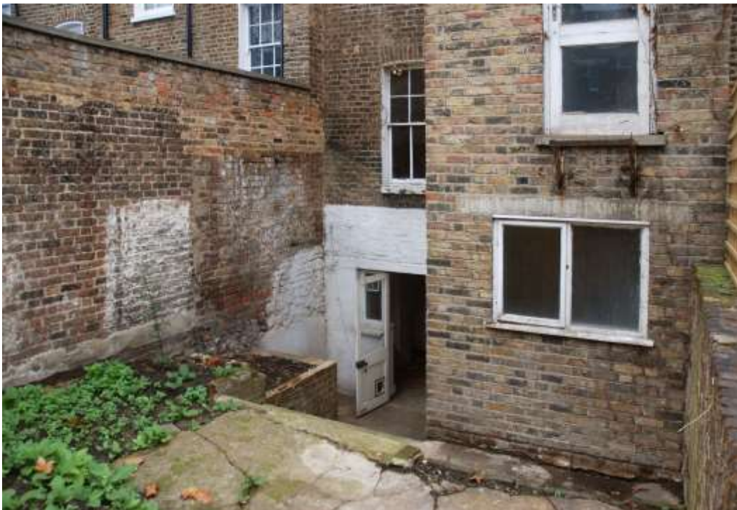
Fig.27: A further view from the southern boundary, the recent extension in foreground. To the rear is the area of the former outbuilding, now occupied by a modern brick retaining wall adjoining the steps
