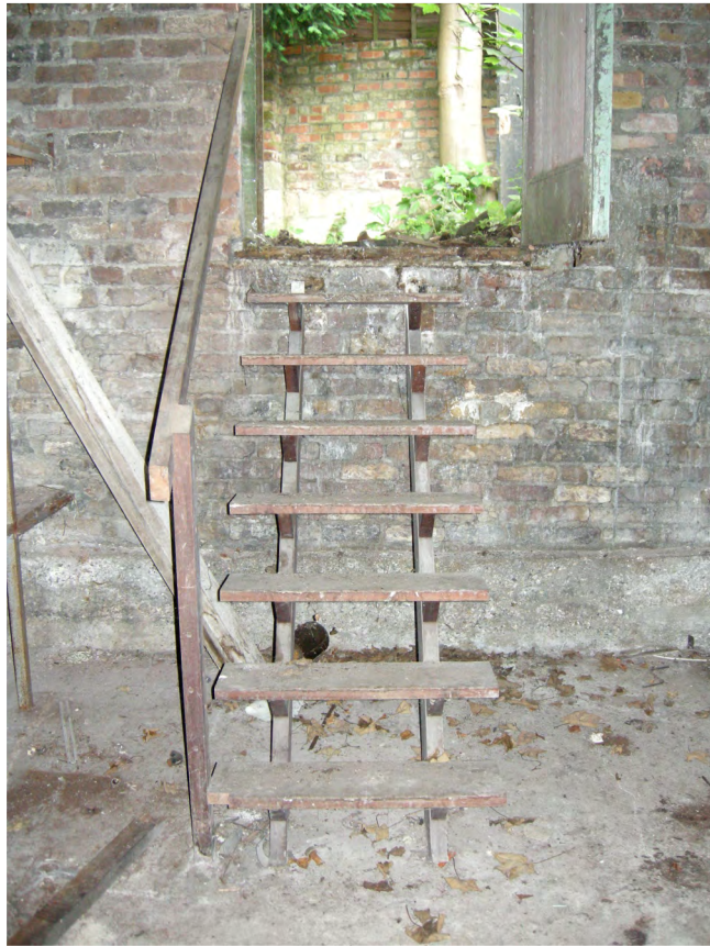
Fig 15 View from north-east of south-west wall of store in north corner of 6 Streatley Place showing depth of floor below ground level (MOLA Photo 16.06.2014)
