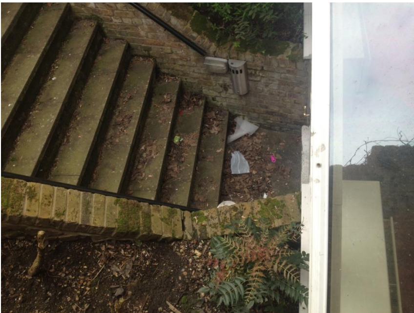
Photo 03 – 104 Albert Street–Garden level lower than 106 Albert Street garden level.
