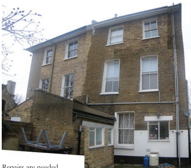
Repairs are needed
