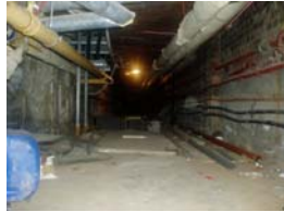
12. Void within boiler house
