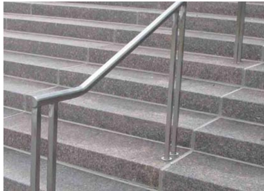
Stainless Steel Handrails to steps
