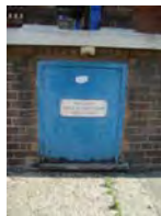
92. Old filling point for AST's
