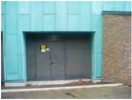
120. Electrica sub station
