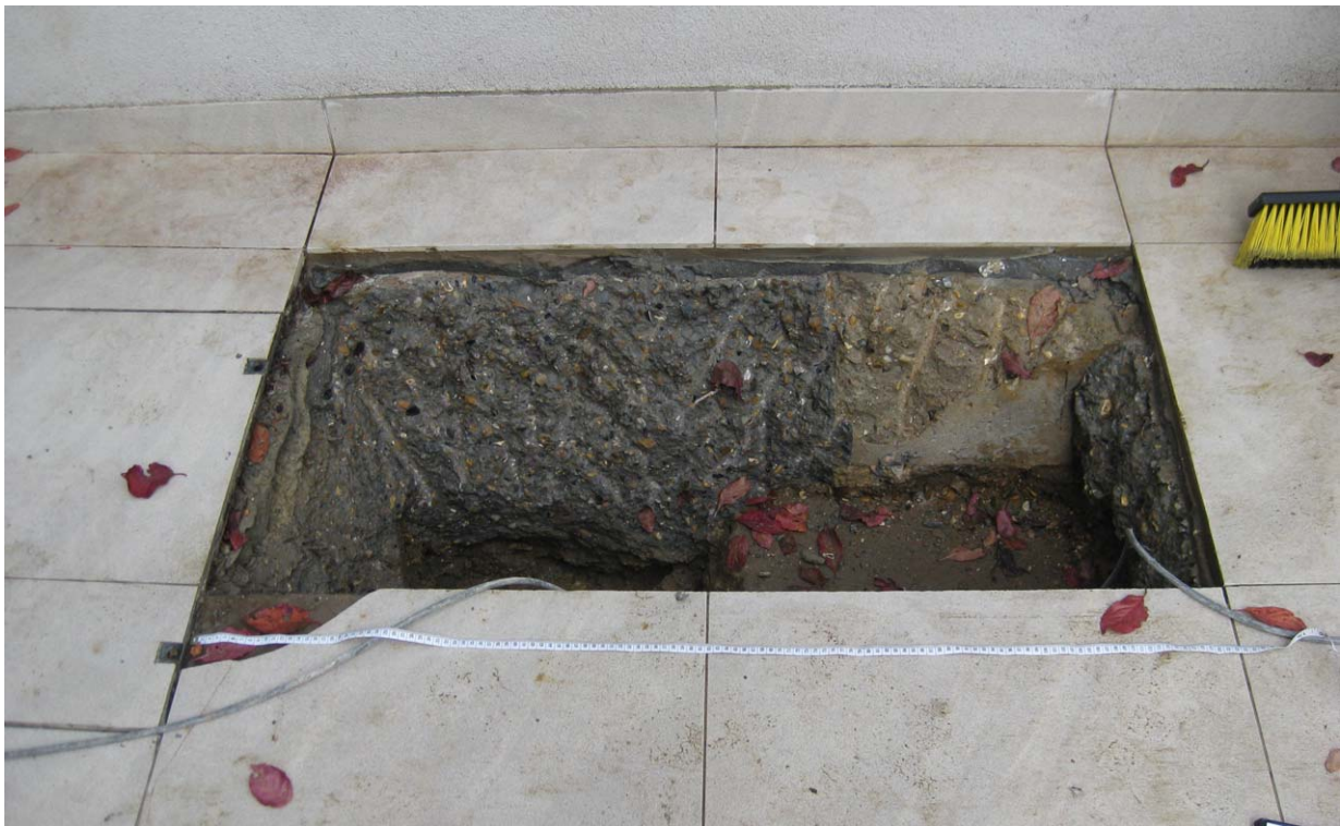
Photograph No. 08 - Trial Hole No. 1 - The trial hole demonstrates the depth of concrete sub-base beneath the existing paving area. The existing topsoil / subsoil layer is located at a significant depth below the paving surface.
