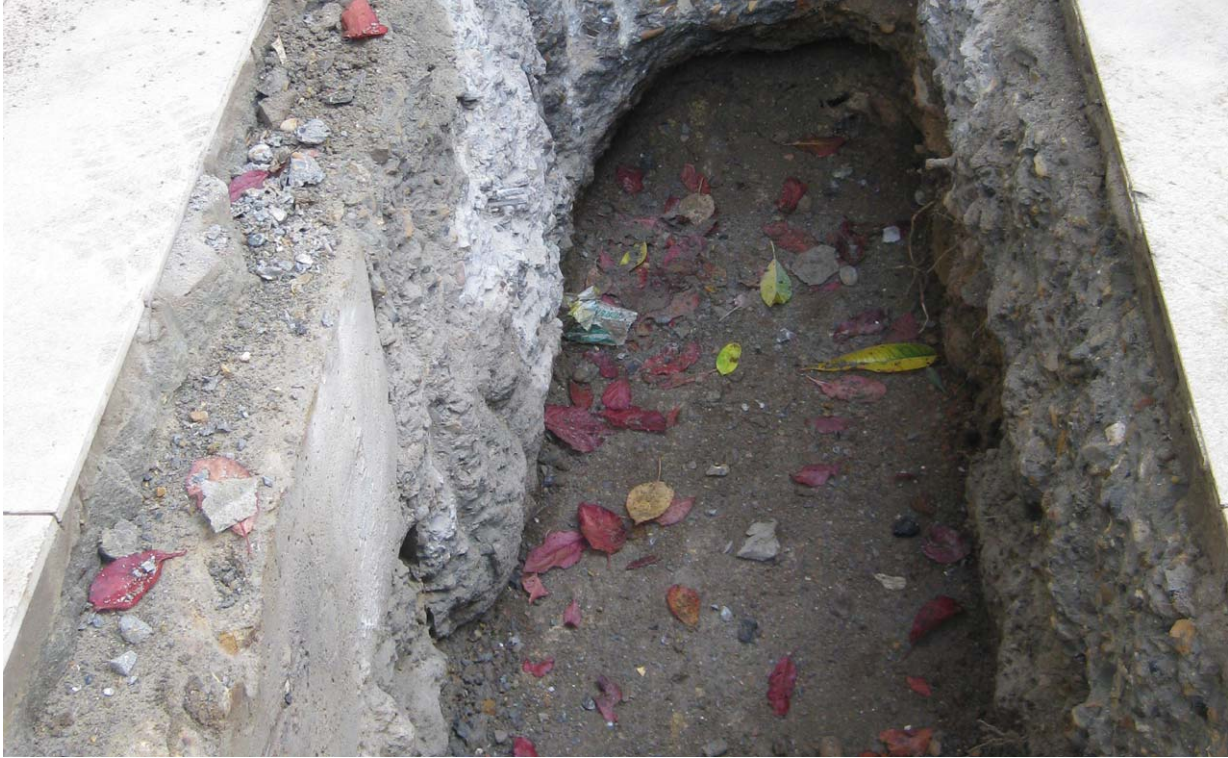
Photograph No. 11 - Trial Hole No. 2 - The trial hole demonstrates the depth of concrete sub-base beneath the existing paving area. The existing topsoil / subsoil layer is located at a significant depth below the paving surface.
