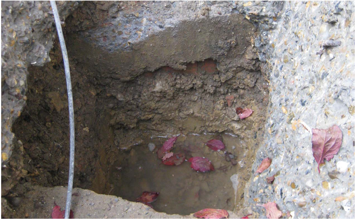
Photograph No. 09 - Trial Hole No. 1 - The trial hole demonstrates the depth of concrete sub-base beneath the existing paving area. The existing topsoil / subsoil layer is located at a significant depth below the paving surface.
