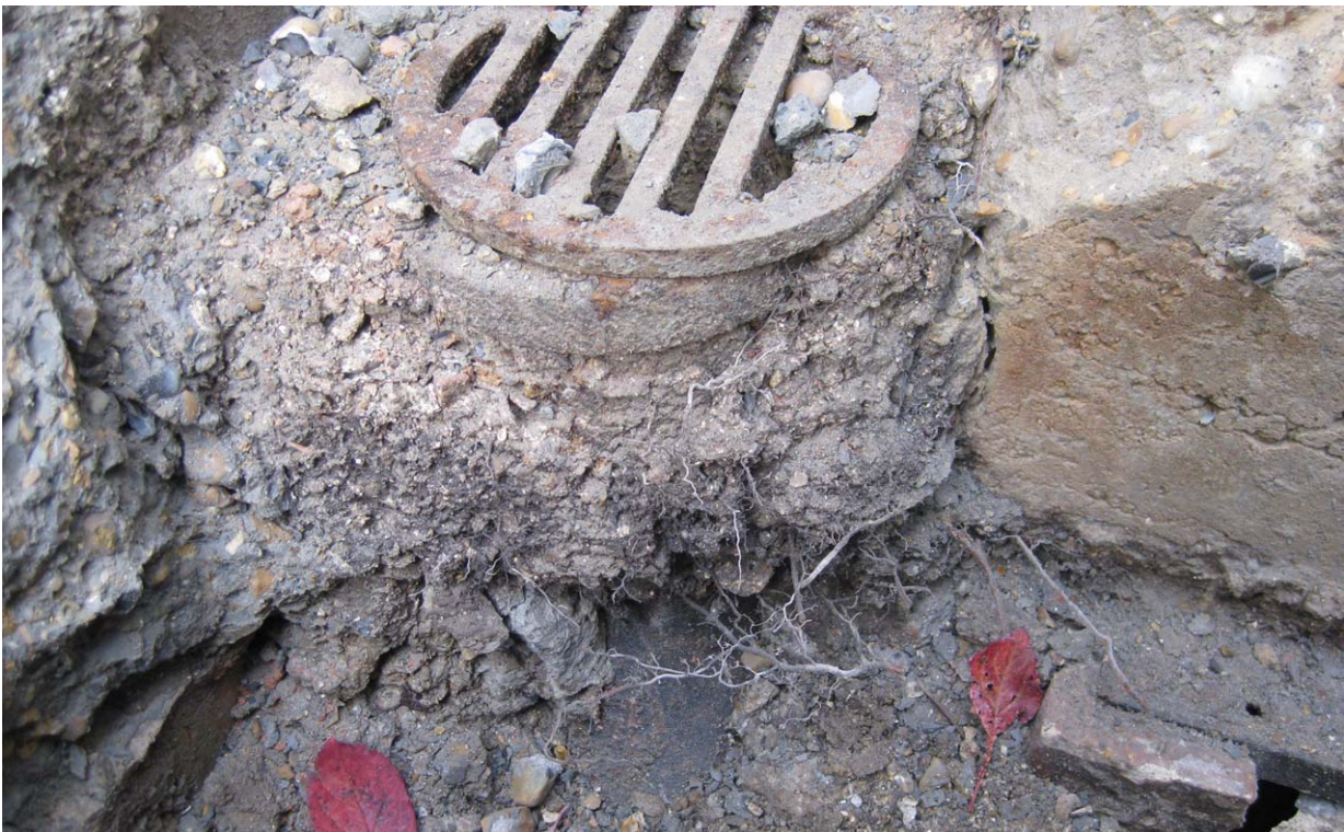
Photograph No. 12 - Trial Pit No. 2 - There were no significant tree roots found within the trial hole, only small fibrous tree roots beneath the concrete sub-base layer of the adjacent plum tree, surrounding the drain cover.
