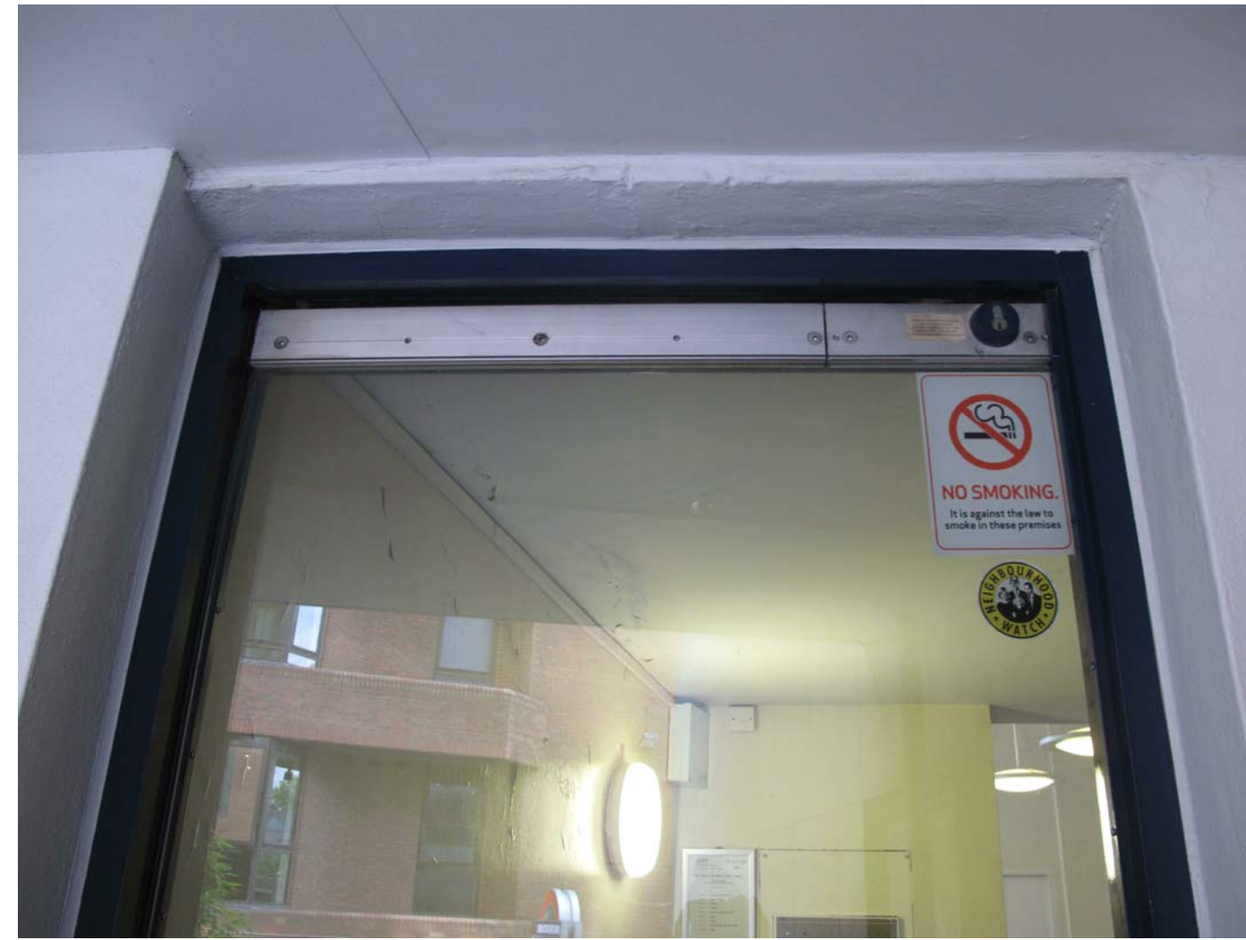
3 Existing steel frame door to be replaced
