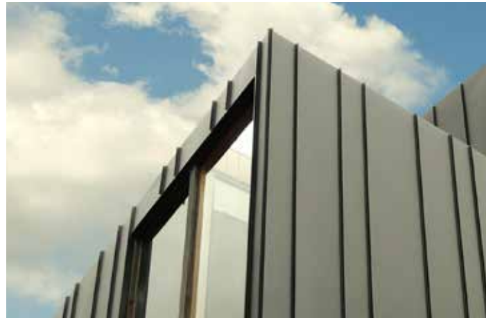
A BLACK ZINC TO MIMIC THE SLATE TILES USED ELSEWHERE IN THE AREA
