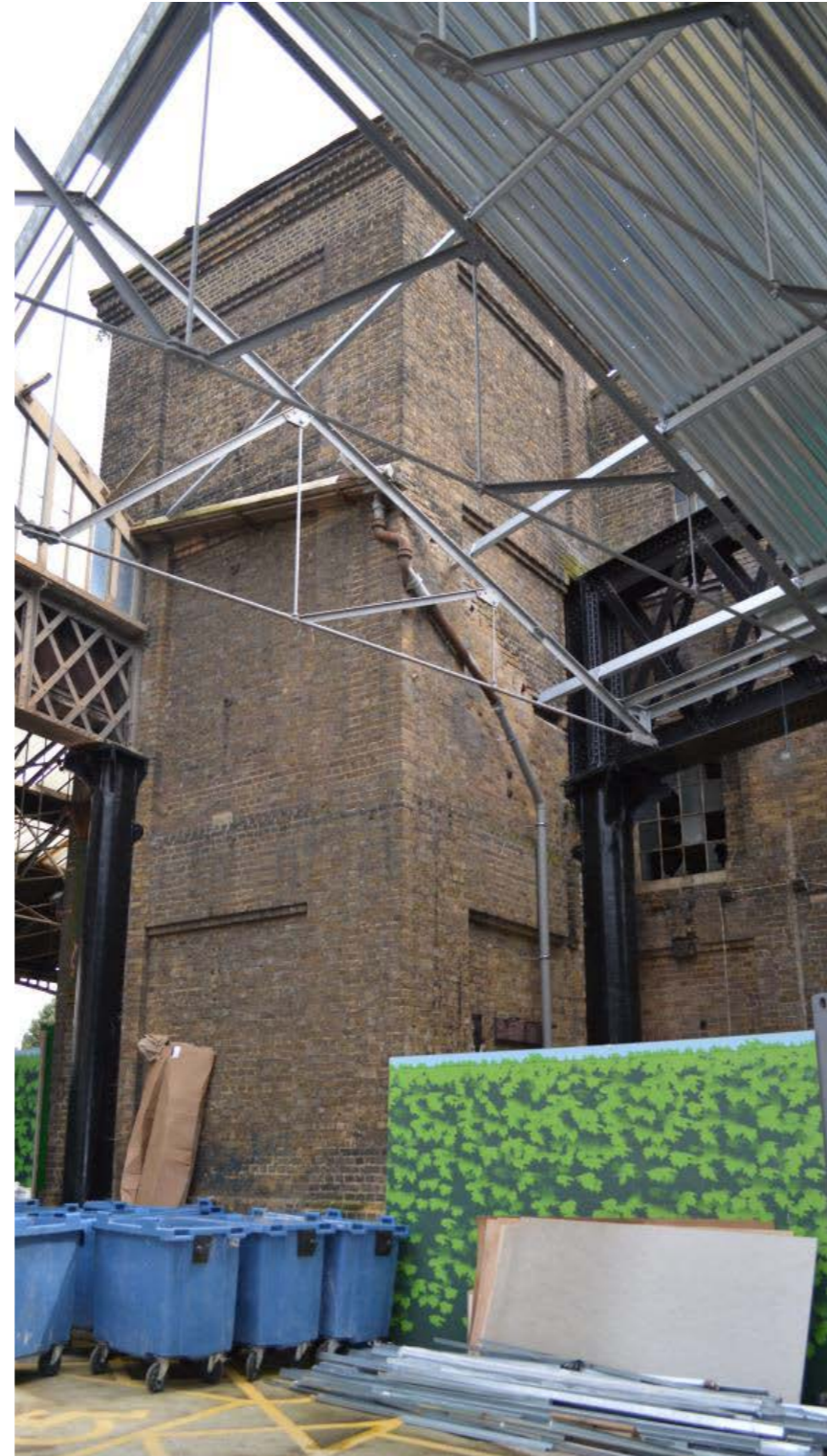
Accumulator Tower - Exterior View
