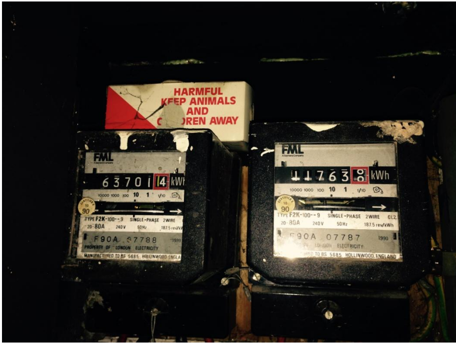
Figure 6: Separate Utility meters
