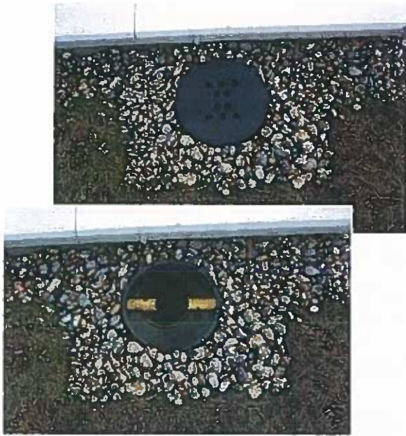
▲ Bauder inspection chamber with surrounding pebble vegetation barrier
