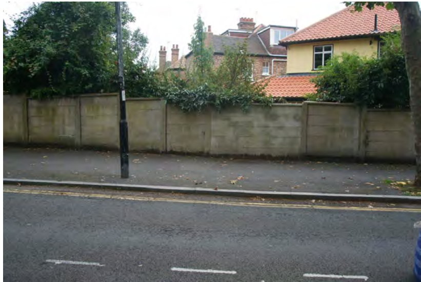
Fourth section of the wall, including the section made from rendered blockwork.
