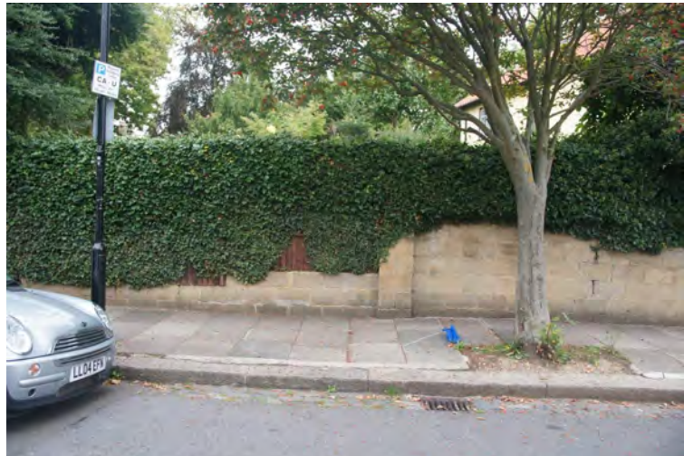
Second section of the wall, showing wooden palings on top of blockwork
