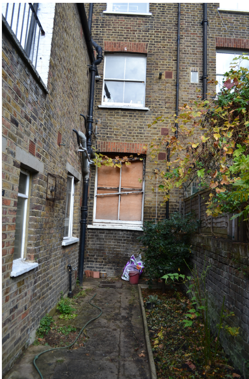
View of sash window to rear reception and area for proposed extension.
