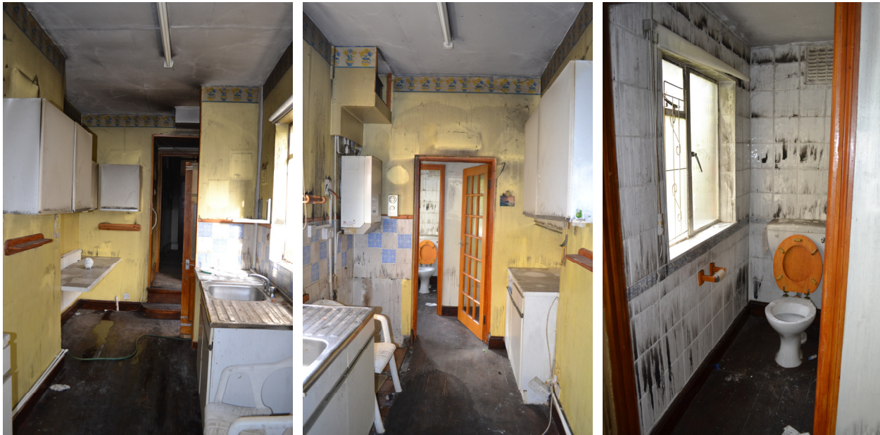
Fire damage in the kitchen and bathroom.
