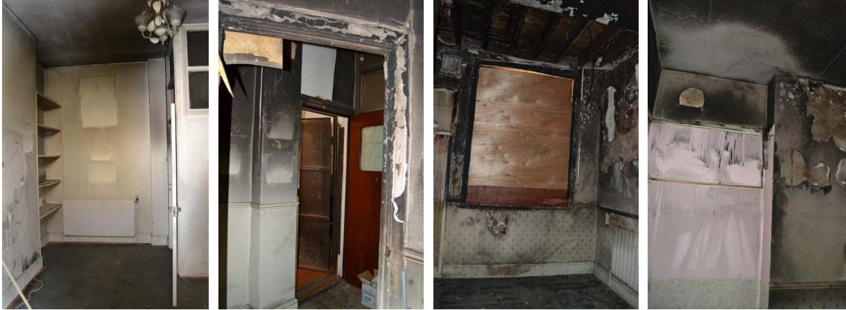
Fire damage in the front sitting room and rear reception room.
