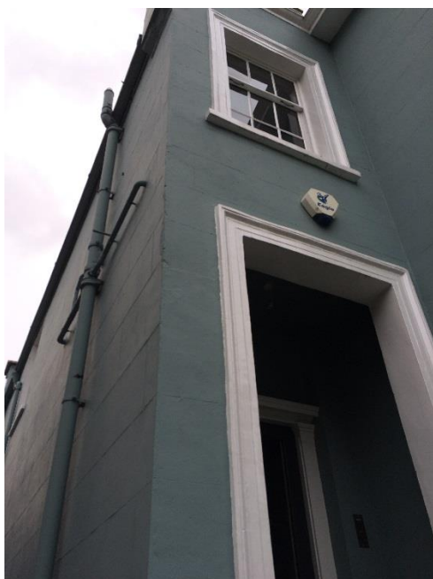
Existing pipework to side elevation which will be used. No new pipe work needed
