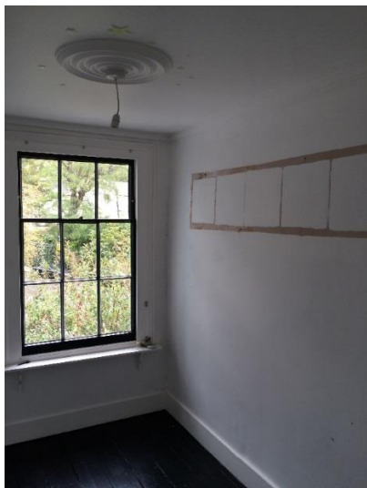
Reinstatement of former opening at first floor to provide access to new bathroom
