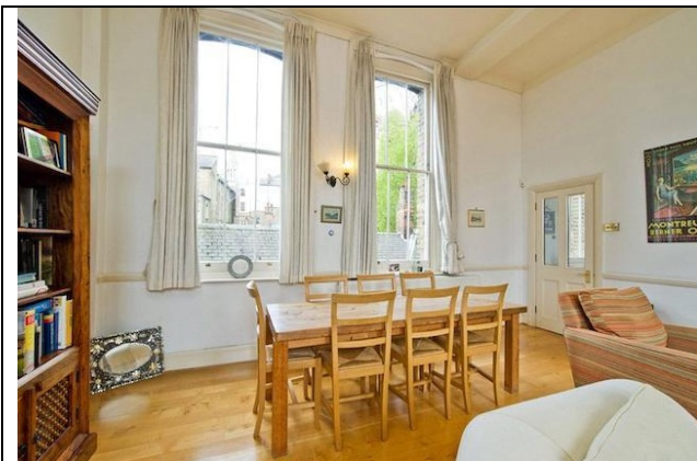
View of 'existing' Reception / Dining Room. Note - new ceiling is built lower than head of window and so is detailed around the window with no cornice etc.
