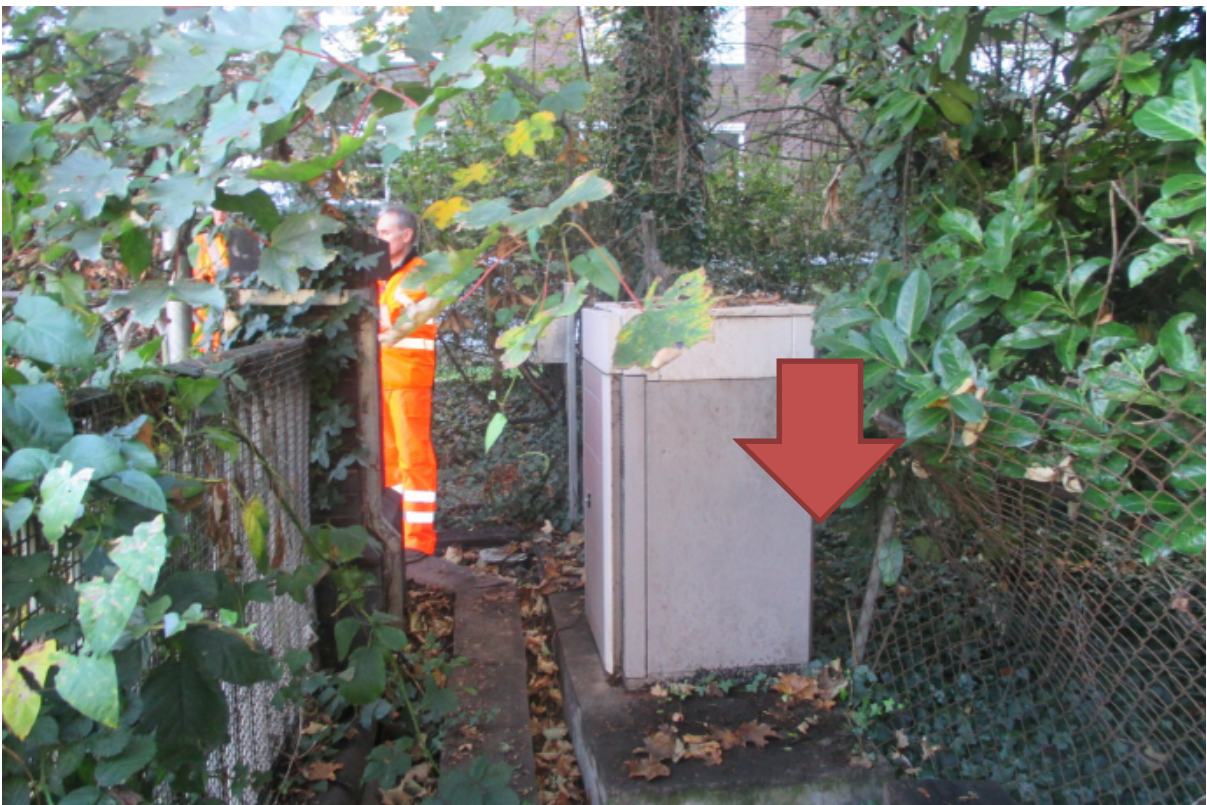
1.3 A second cabinet will sit next to this one, where the red arrow points
