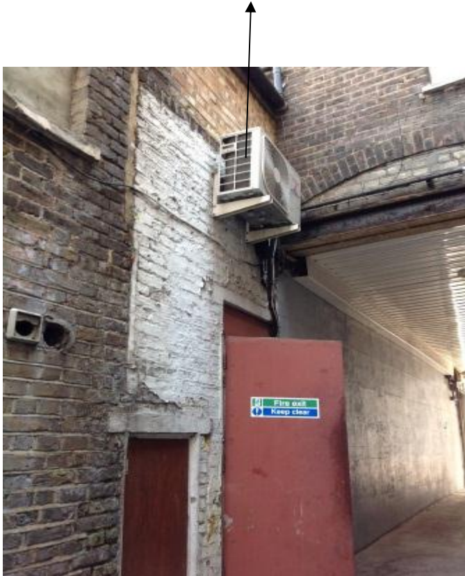
Photo 2- Side elevation- AC unit to be removed
