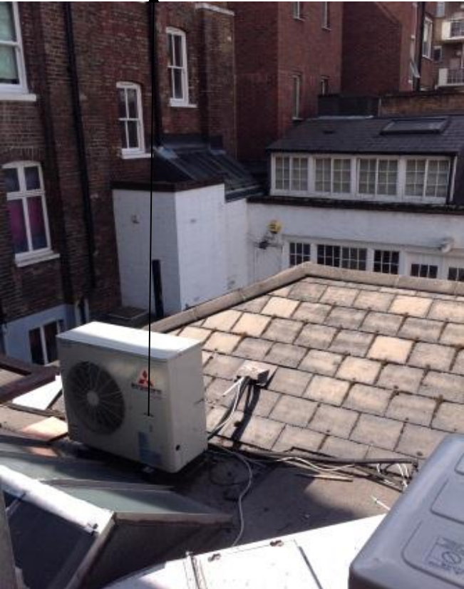
Photo 4- Ac unit on flat roof of outbuilding
