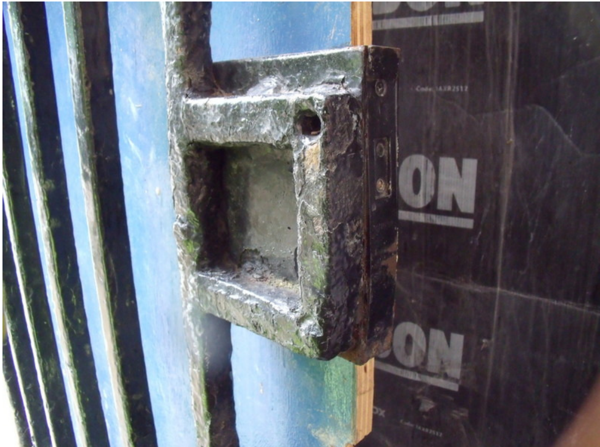
Close up of lock on gate showing original lock frame and newly added modern lock on the inside.
