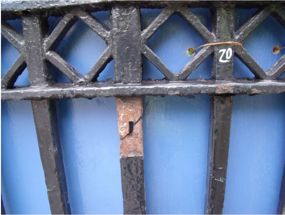
Close up of break at Paling 19, where back stay should be.
