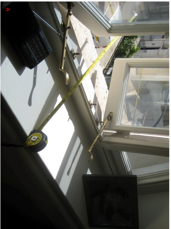
A Photographs displaying typical existing upper storey window ironmongery. To be retained
