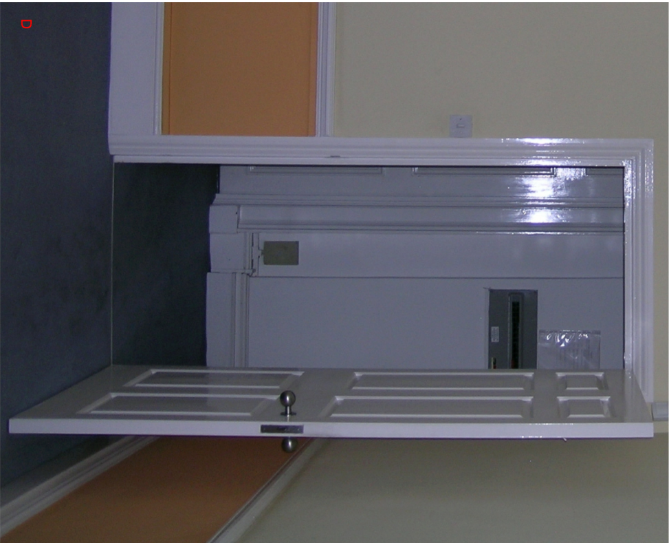
photographs displaying typical existing door handles - upper floor doorways
