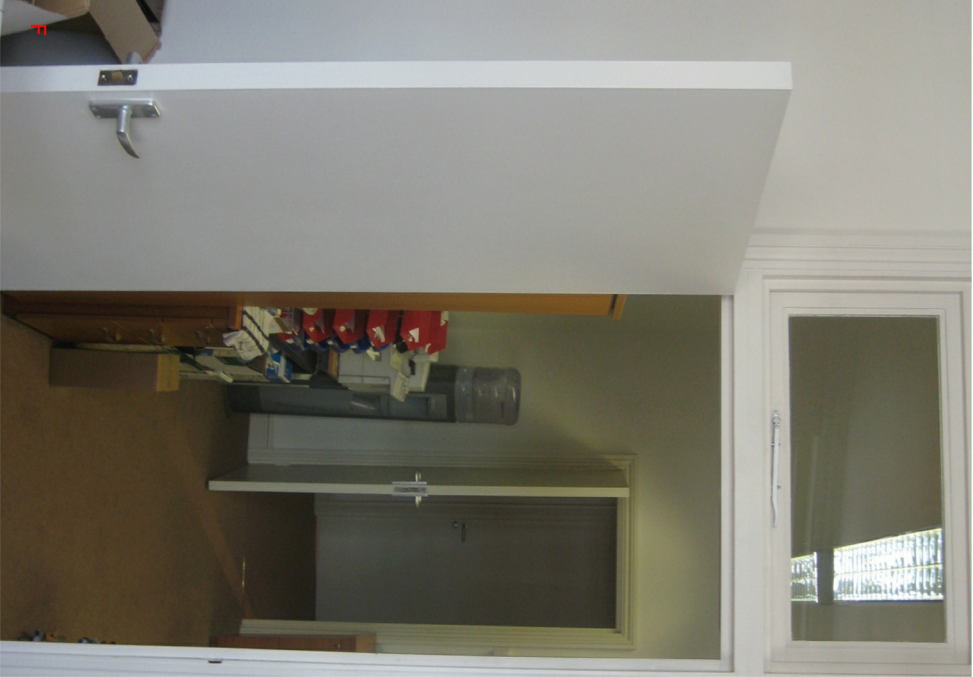
photographs displaying typical existing door handles - upper floor doorways
