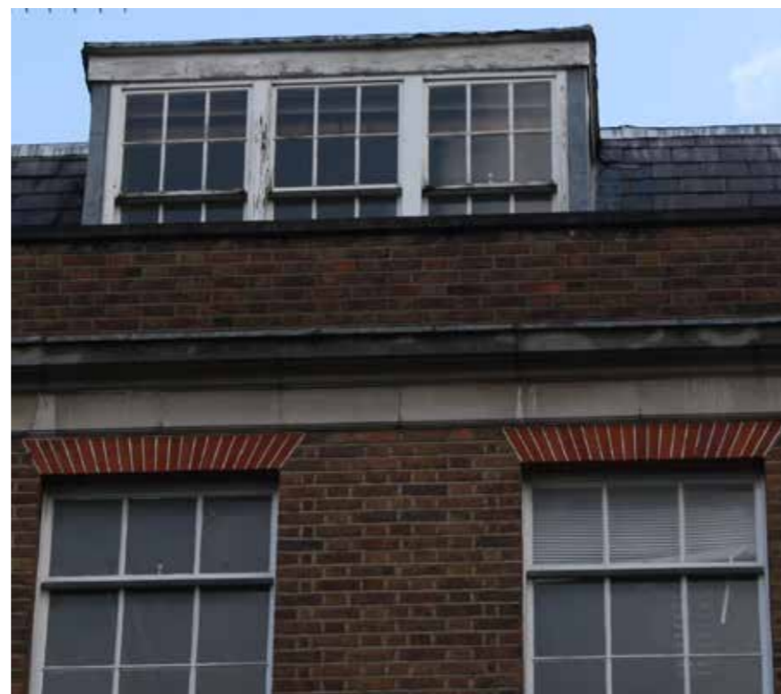
TIMBER SASH WINDOWS TO FRONT IN POOR CONDITION
