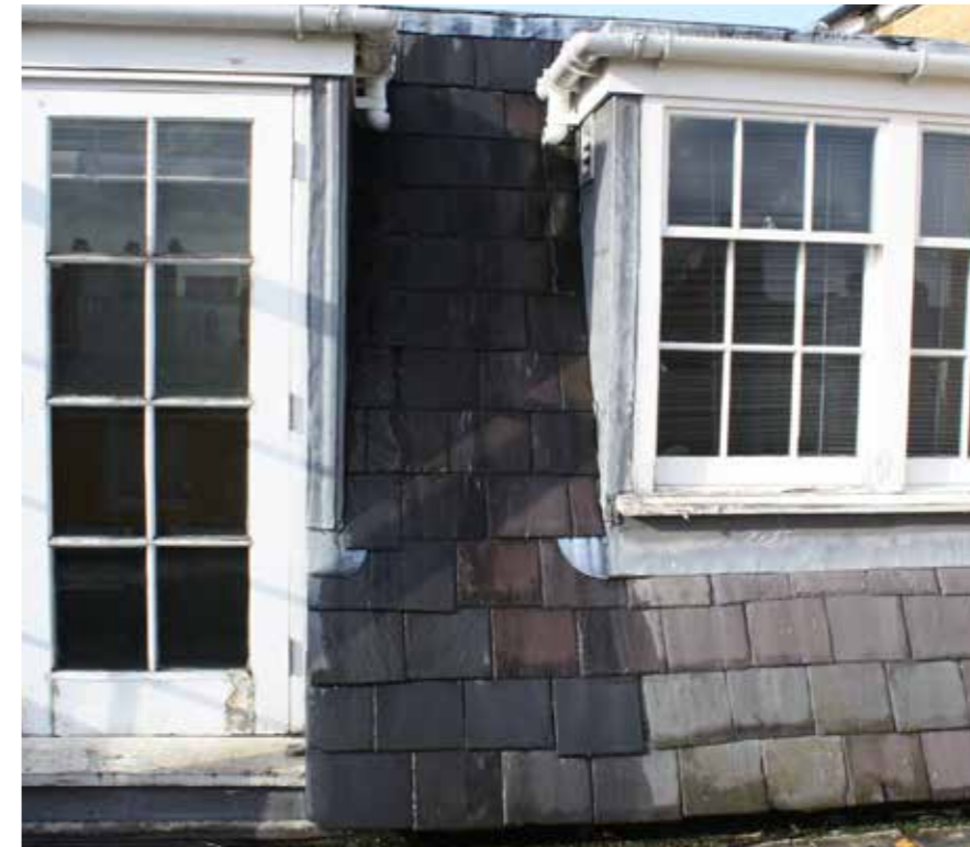
DILAPIDATED REAR MANSARD
