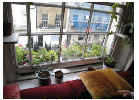
living room - defective sash window
