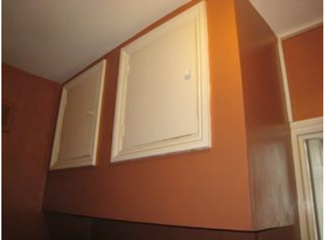
high level water tank
