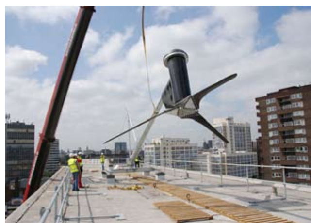
A building-mounted 6kW Proven wind turbine
