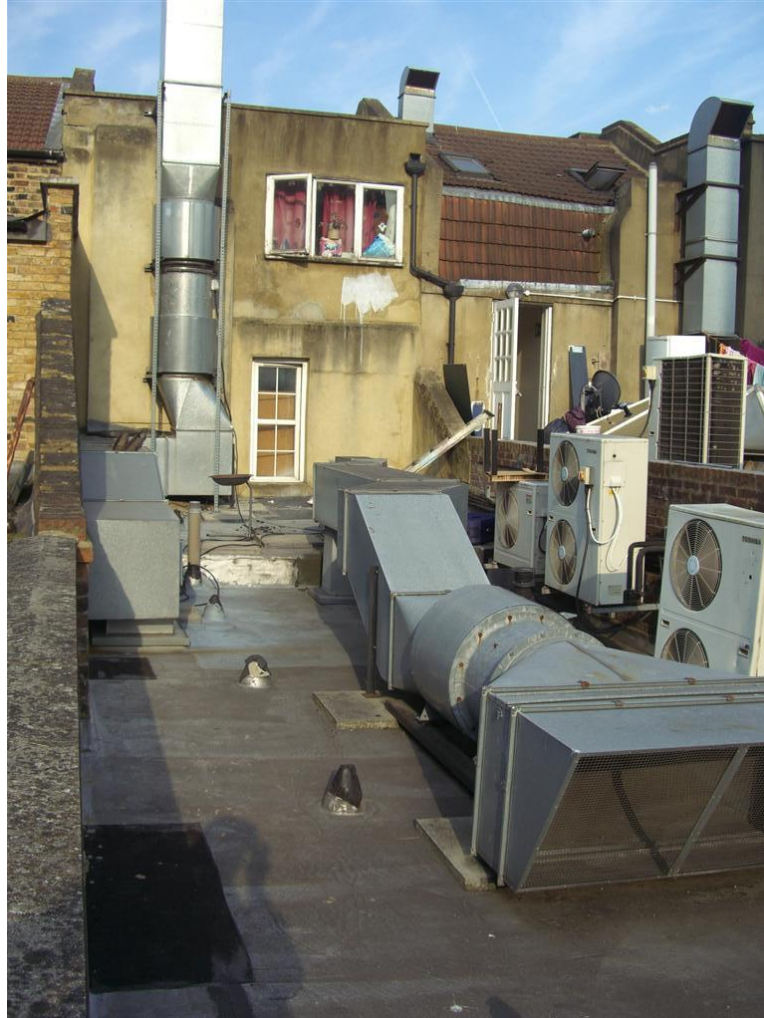
View of the existing supply and extract ventilation systems on the first floor roof of 239 Camden High Street.
