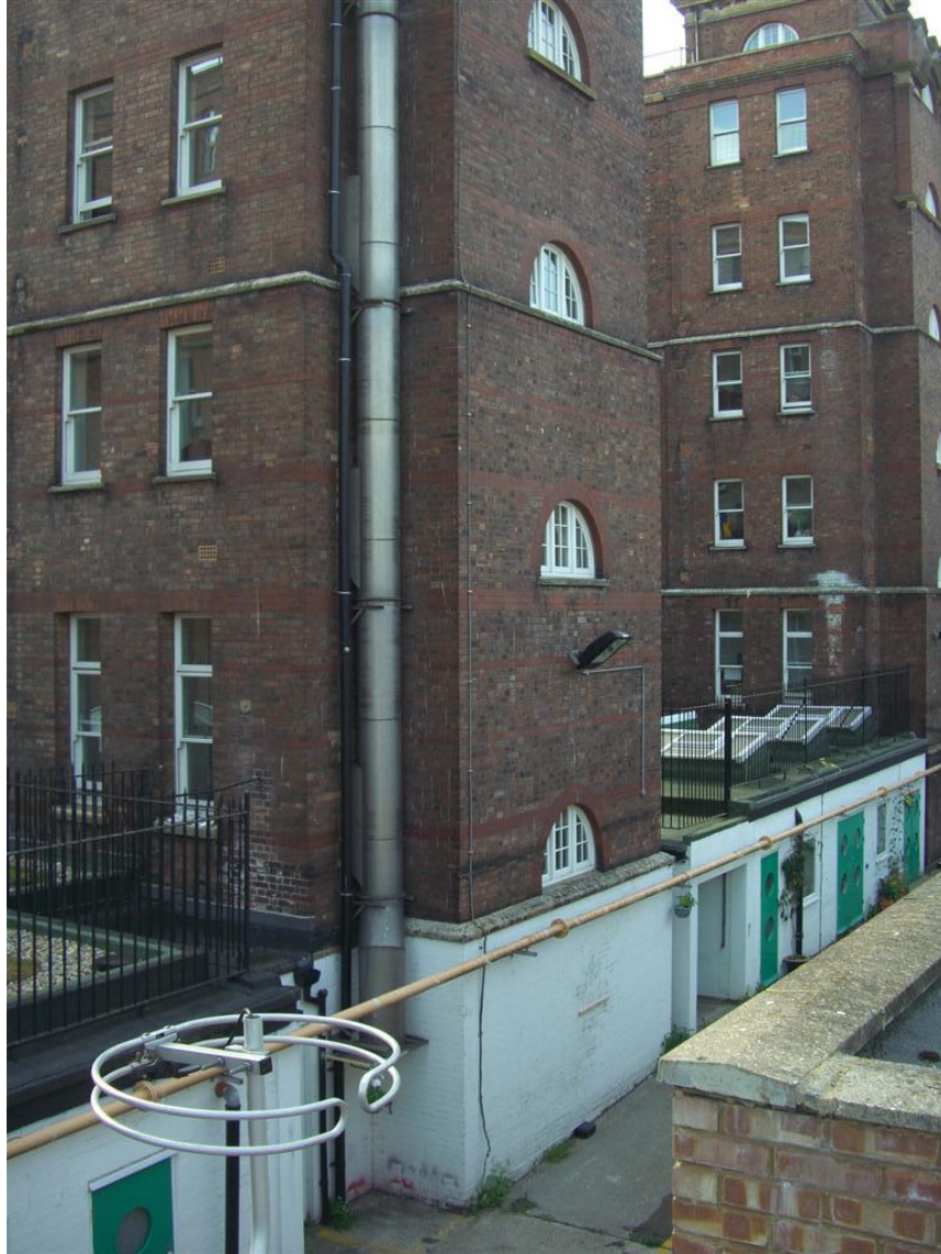
A view looking towards Arlington Conference Centre from the first floor roof of 239 Camden High Street. Part of Arlington Conference Centre is residential.
