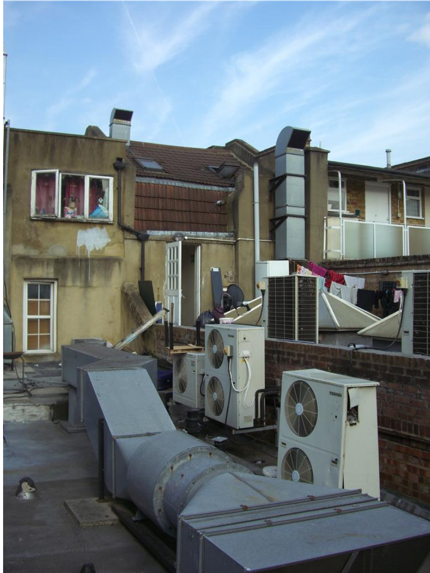
View of the existing fresh air ventilation system and AC condensers on the first floor roof of 239 Camden High Street. The nearest AC unit is redundant; the two AC condensers furthest to the right are on the roof of 237 Camden High Street.
