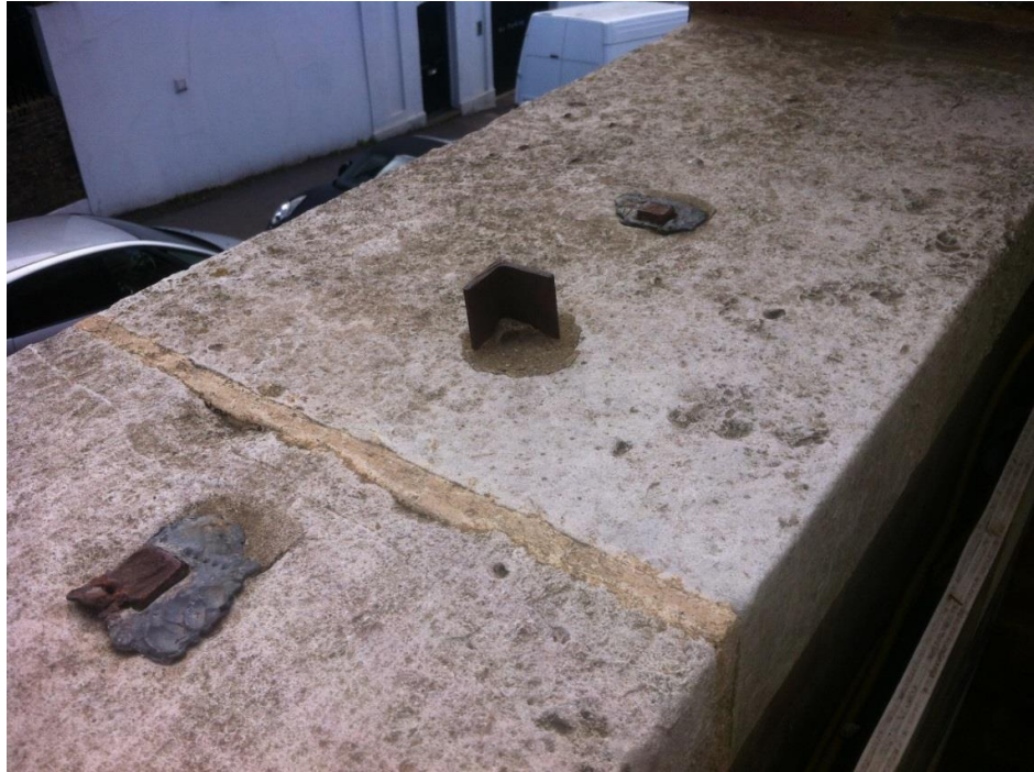
5. An example of previously poorly fixed metalwork to stonework elsewhere on the site.
