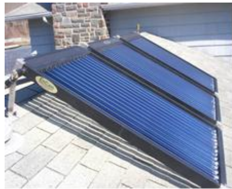
Figure 9: Example of Solar Thermal System
