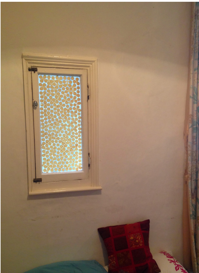
Interior view of the existing bedroom window to be replaced at No. 17 Belsize Park Gardens
