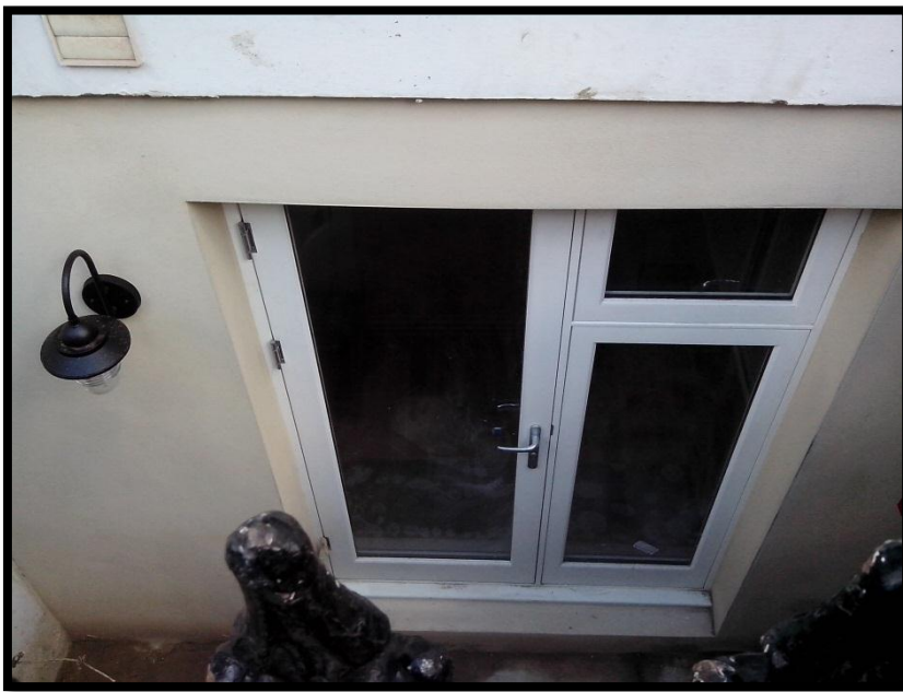
Photo 5: View to new timber framed doors at lower ground floor (with new timber doors shown)
