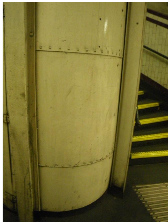
Figure 4: Photograph of the metal 'tube' running down the centre of the spiral stairs that screens existing services. Outlet box to be located facing out of this 'tube'.
