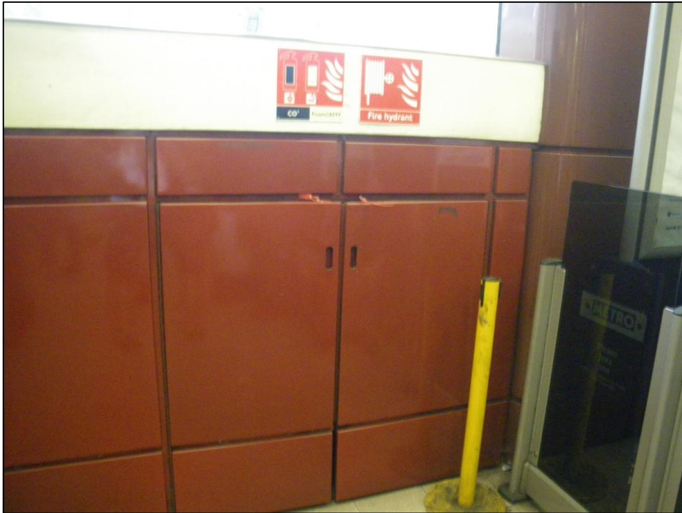
Figure 3: Photograph showing the existing fire hydrant at ticket hall level.
