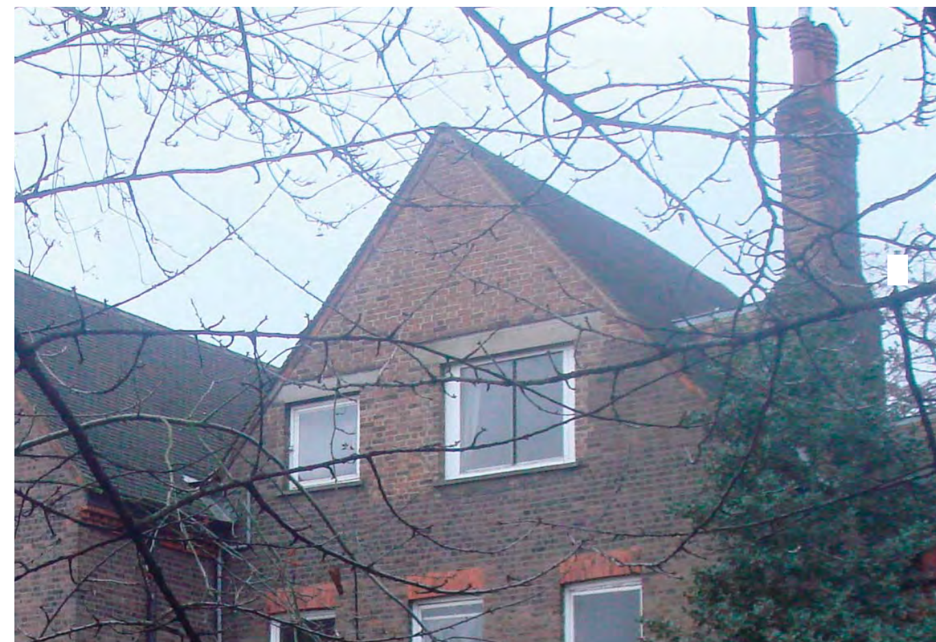
Poorly proportioned windows, extensive non-original poorly matched brickwork and concrete lintels
