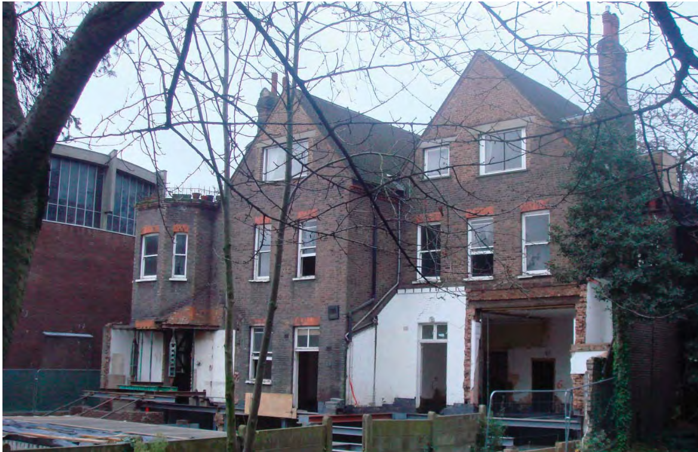
The rear of no.2 in December 2011, with basement excavated and steel frame in place
