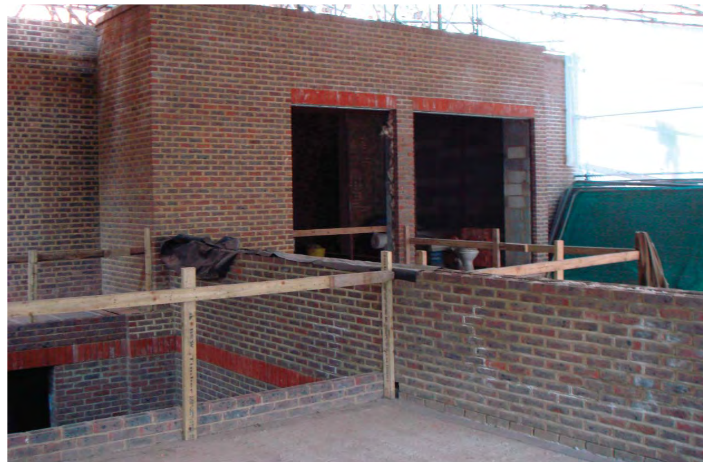
Current status of the site - showing the most complete area of work at the rear
