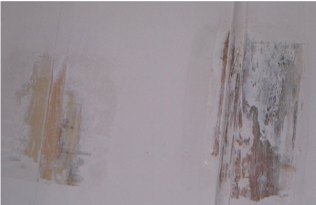
2 No. Paint investigations into original panelling on west wall of ground floor rear room
