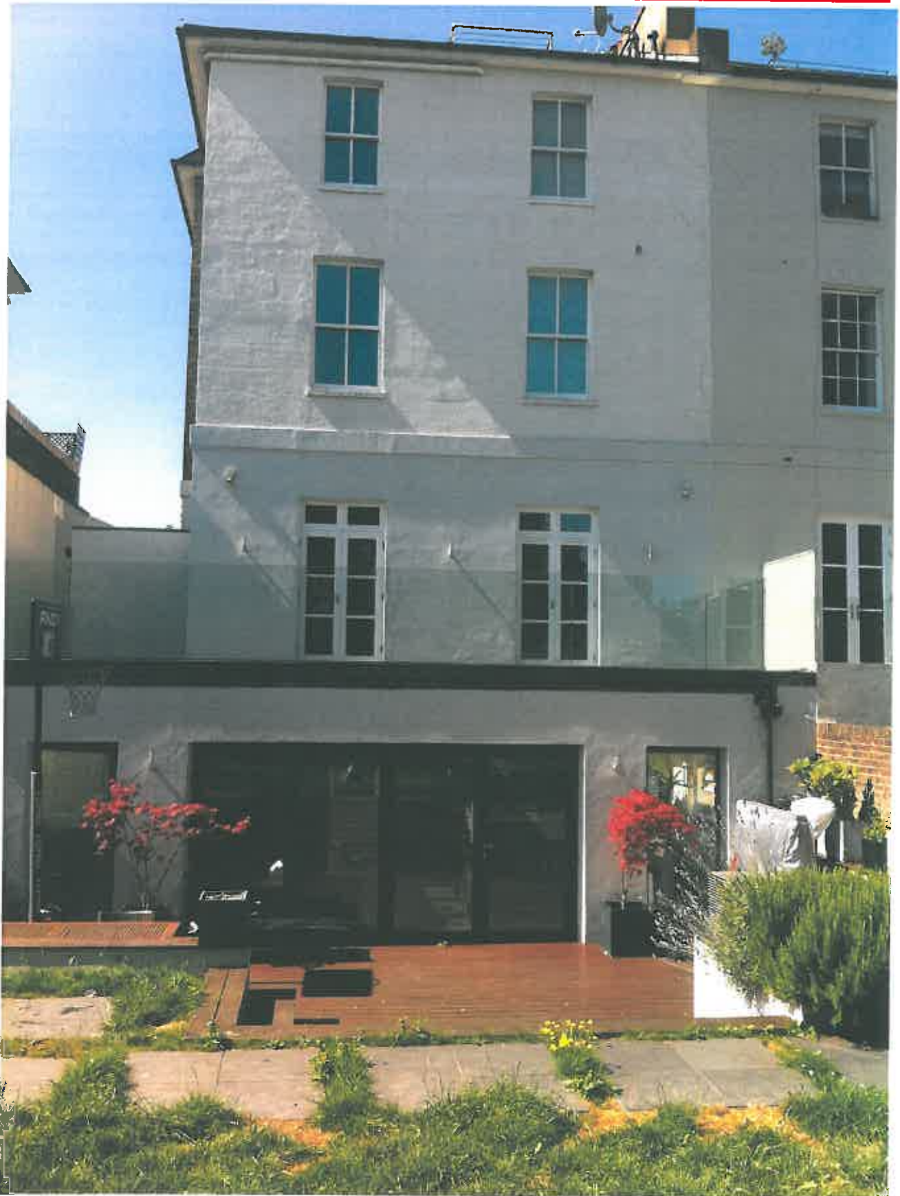
Photo 4 - View of rear of house showing party wall with No170 (right of frame)
