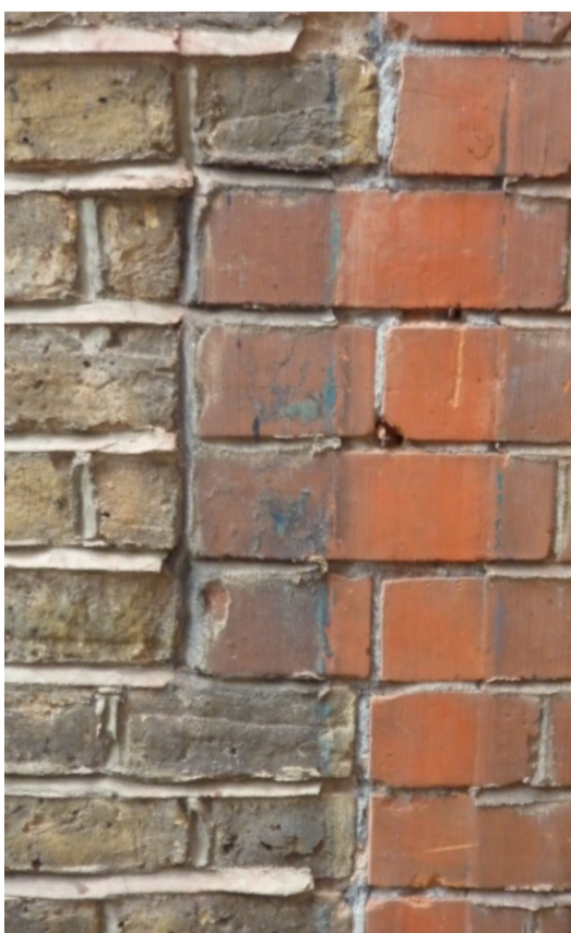
poor workmanship to mortar beds
