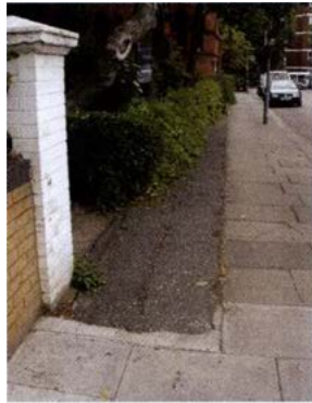
5. uneven pavement, Elsworthy Road Before council improvements
