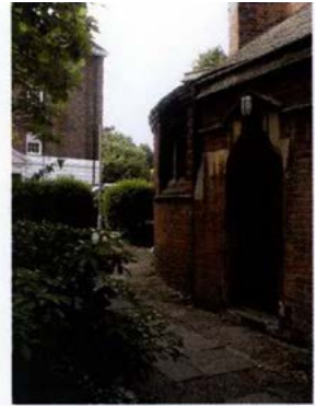
6. Uneven pavers at east entrance Before Construction of the St Mary Centre
