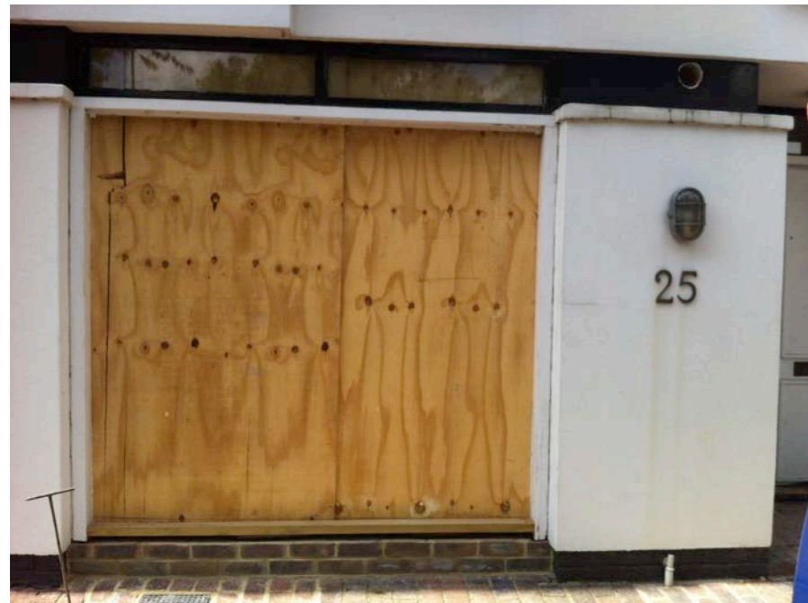
No 25. Garage boarded over
