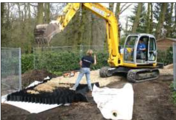
Photo 11: Cellular products are a very effective means of providing ground protection where heavy vehicle use is expected. Here, it is being used to temporarily widen an existing road, to be removed once the construction is finished.
