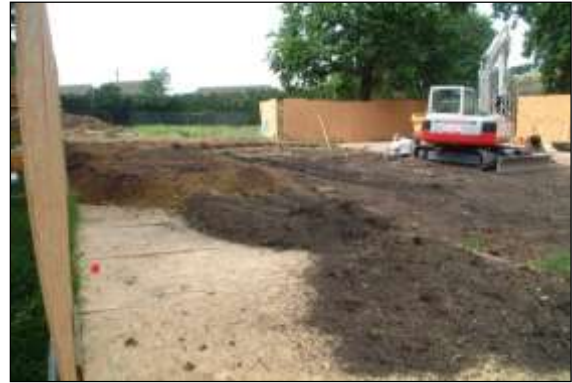
Photo 8: Spreading soil excavated from footings is an effective way of buffering the plywood surface from the wear of light vehicles.
