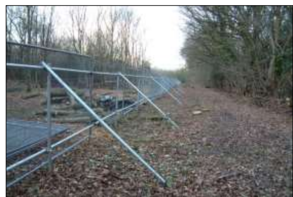
Photo 2: Heras fencing wired to scaffold braced posts is a robust and effective interpretation of the BS specification.
