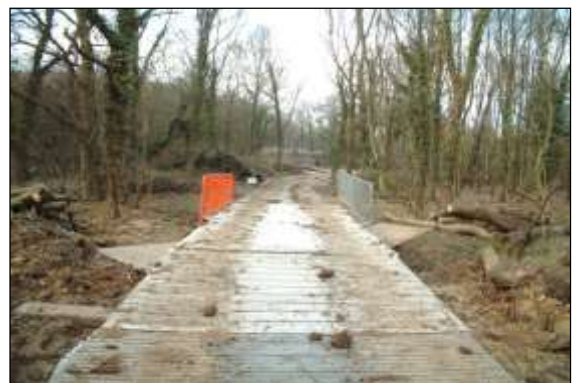
Photo 12: Custom designed sectional tracks can be joined to support very heavy traffic use through sensitive areas.
