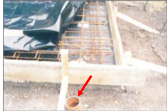
Photo 43: This reinforced base slab for a double garage has drainage provision (red arrow) beneath the structure to redirect roof runoff to supply roots with water.
