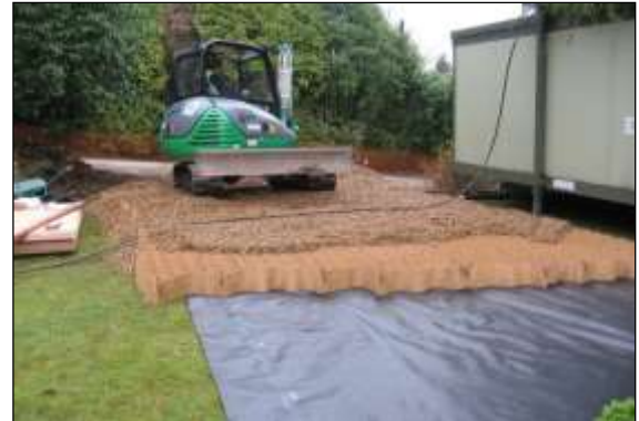
Photo 25: The stone-filled cells spread the load of traffic and the geotextile membrane on the ground prevents migration of the stone into the soil profile.
