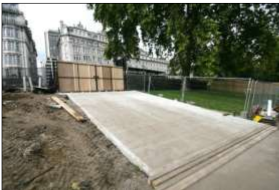
Photo 30: This temporary access for heavy construction traffic on the outer edge of a RPA is a concrete slab cast above ground level and will be removed when the project is completed.
