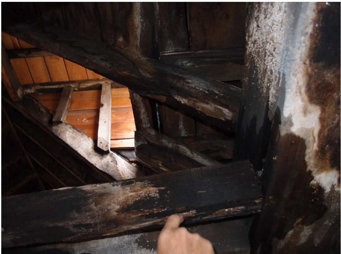
Figure 15 – LHS roof beam underside gully showing signs of decay
