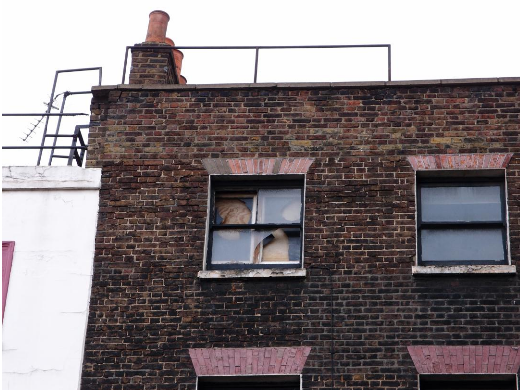
Figure 2 – Front Elevation upper floor window head & displaced coping brickwork
