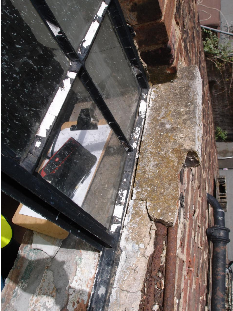
Figure 25 – Typical metal Crittall window and broken concrete cill
