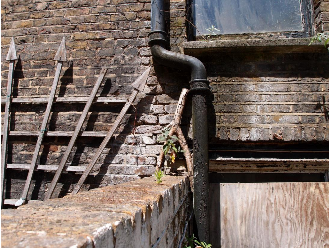
Figure 9 – Rear extension brickwork affected by plant growth
