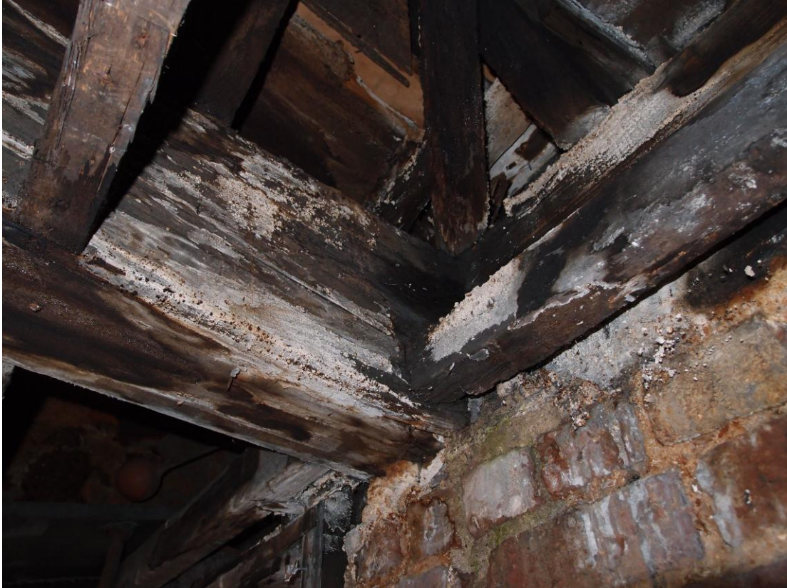
Figure 14 – RHS roof beam underside gully showing signs of decay
