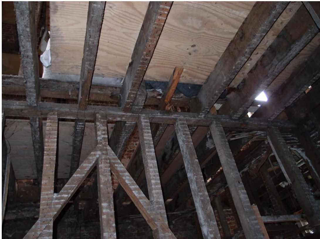
Figure 21 – First floor broken floor joist
