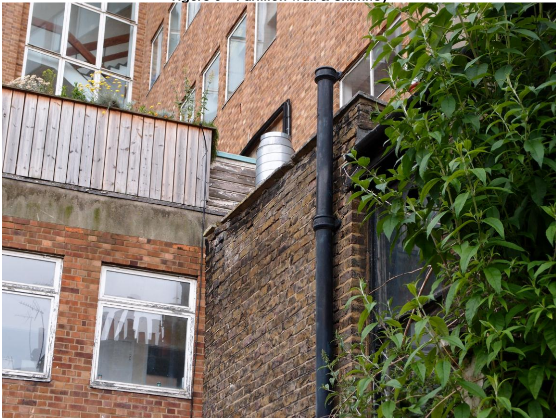
Figure 6 – Rear extension parapet leaning inward
