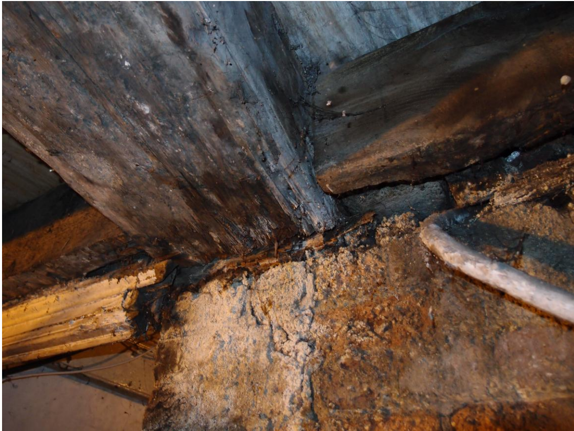
Figure 20 – Large ground floor beamt showing decay
