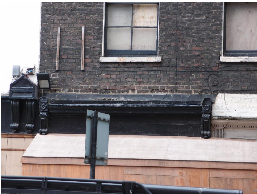
Figure 3 – Front Elevation displaced brickwork at door head
