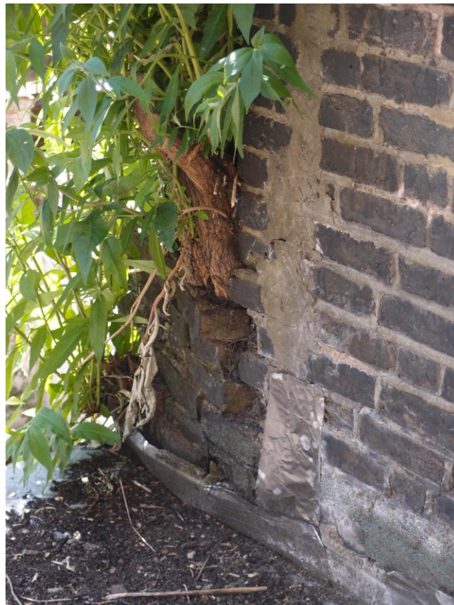
Figure 10 – Rear extension brickwork affected by plant growth
