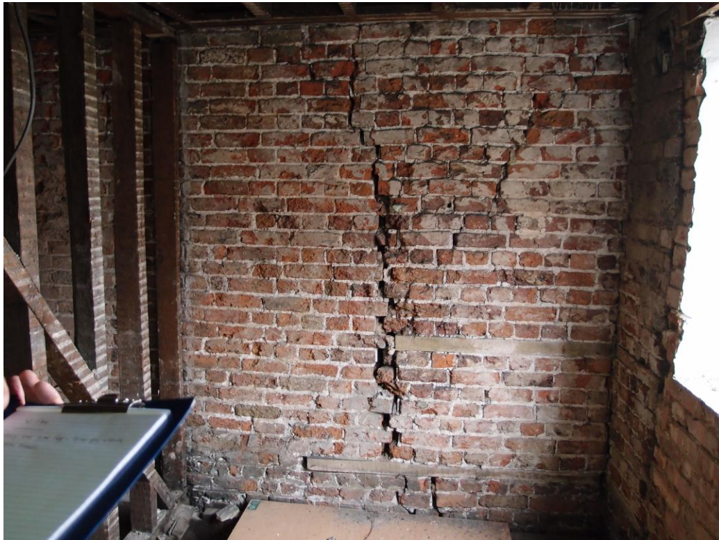
Figure 12 – Internal brickwork upper floor crack at partition wall
