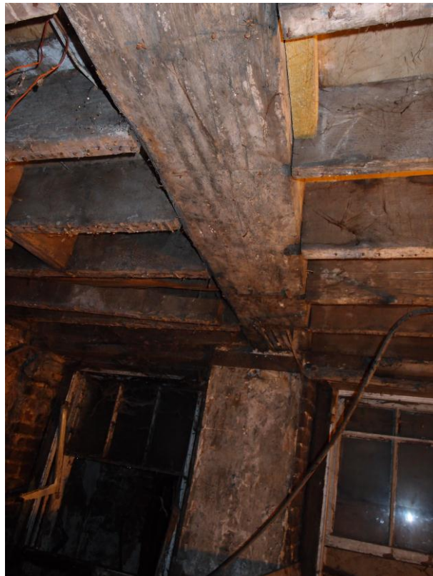
Figure 89 – Ground floor broken floor joist & large floor beam
