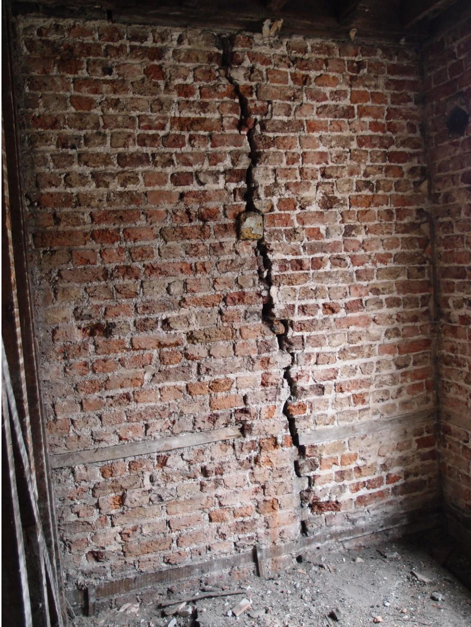
Figure 13 – Internal brickwork second floor crack at partition wall
