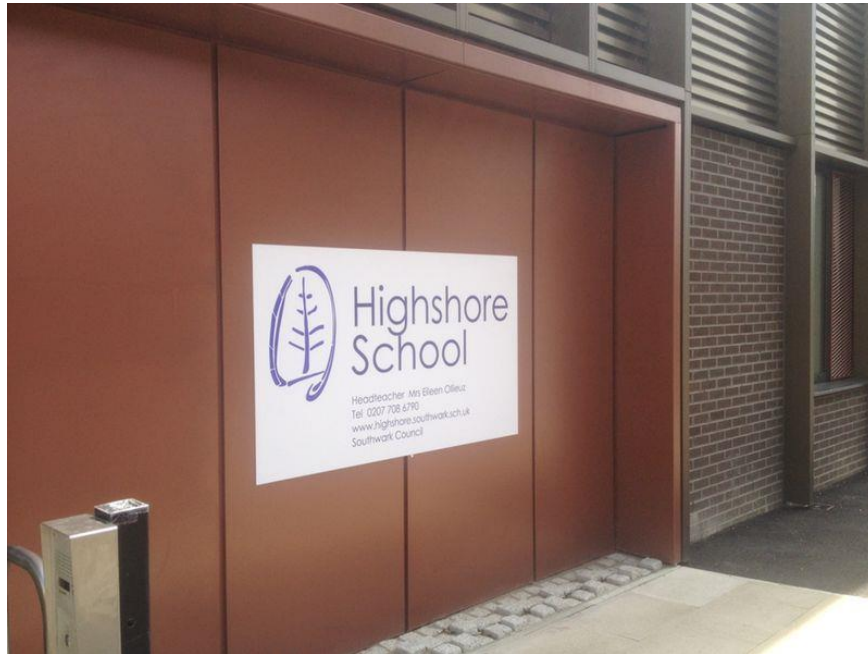
An example of quality powder coated aluminium cladding creating a pleasing palette with brickwork. This new school in Southwark Council has recently been completed.
