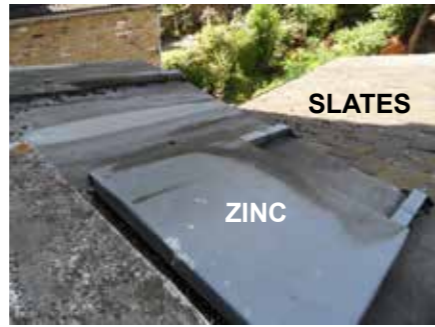
67 Falkland Rd. 2 storey rear projection with a small zinc roof raised over the original slate roof.
