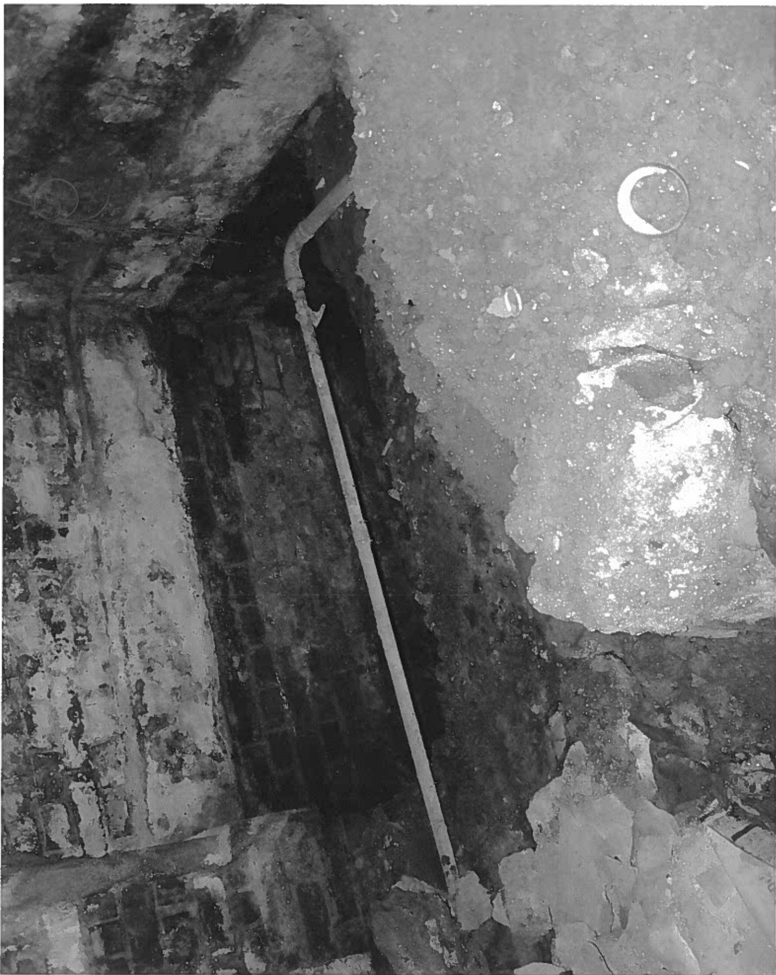
① EXPOSURE OF THE FOUNDATION TO THE FRONT WALL - R.H. CORNER.
