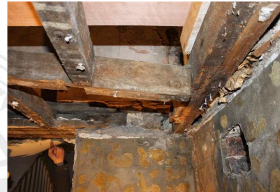
Rotten floor joists. (Woodworm)
